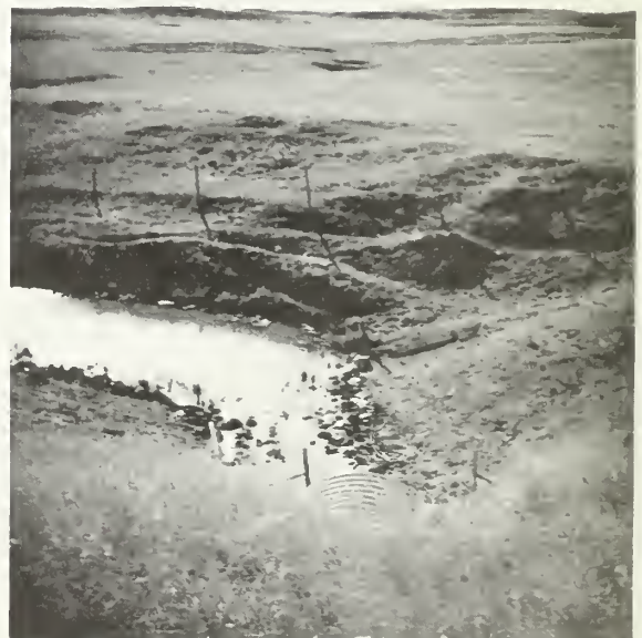
Looking South from SOUTH ENTRANCE Water is seepage from stock reservoir above the pipe.
